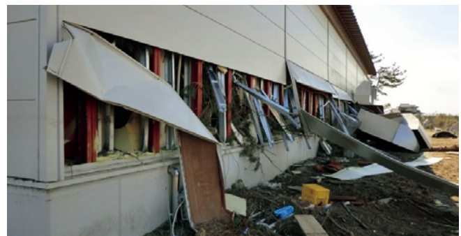
Disaster-struck facilities (Top left) au shop (Top right) au Kamaishi Ryōishi Base Station (Bottom) JIH Sendai Station building
