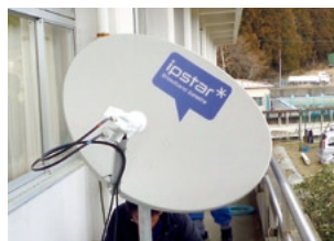
au femtocell antenna using satellite communications (Ishinomaki, Miyagi Prefecture)
