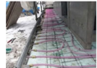
Road heating facilities
