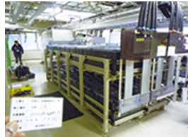
Former 800MHz frequency base station storage battery
