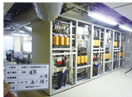
Former 800MHz frequency base station power source
