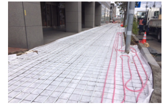
Road heating facilities
